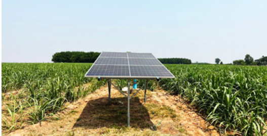
1,800 watts solar panels
