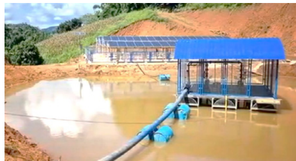
Solar Powered Pumping Stations
